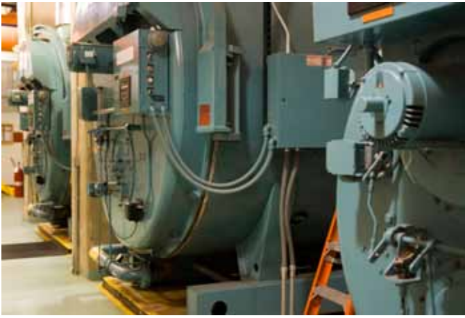
FIGURE 3 Boiler fed by No. 6 fuel oil pump.
